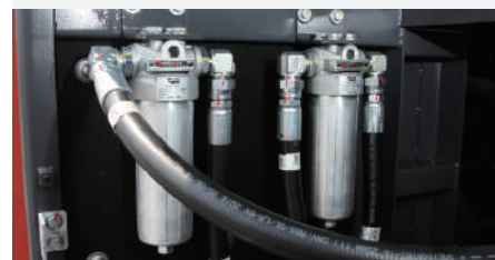
PROTECTED HYDRAULIC SYSTEM
